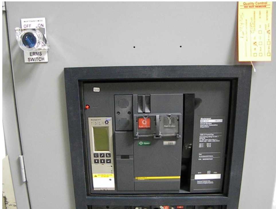
Figure 4: An ERMS-equipped circuit breaker
