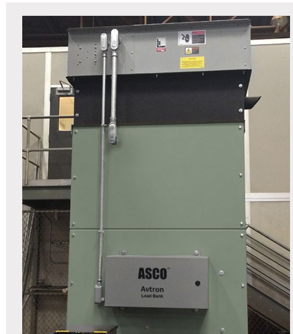
Horizontal Mounted Load Bank shown. (Photo courtesy of ASCO Power Technologies.)
