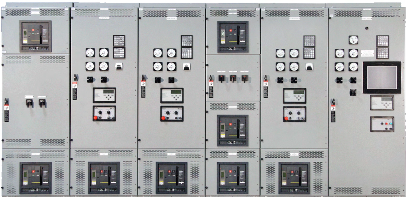
Figure 1: A low-voltage Power Control System lineup
