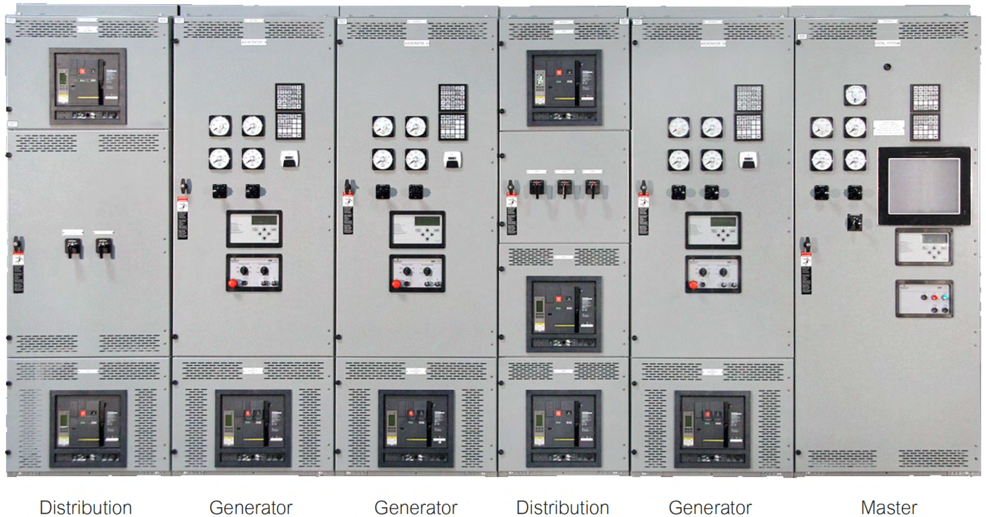
Figure 5: A PCS with a Master Control Section, three Generator Sections, and two Distribution Sections
