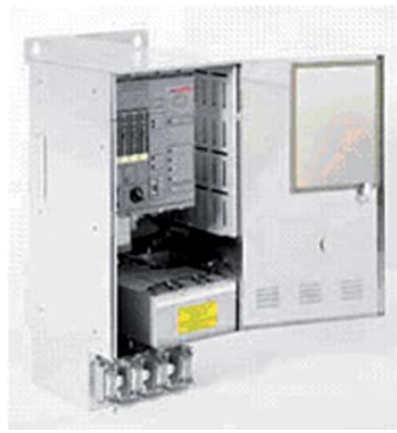
Fig.7- IRTU : integrated remote terminal unit for four feeders
