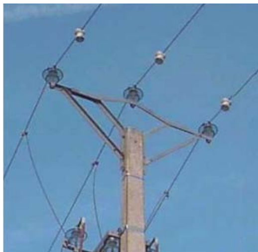
Fig.5 - OH: clip-on fault passage indicators
