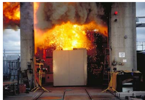
Fig. 3. Medium-Voltage Arc Resistant Switchgear Under Test.
