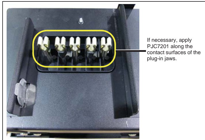
Figure 6: Inspect Plug-In Jaws
