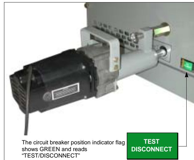
Figure 3: ERD Mounted on the Circuit Breaker Compartment Door (Circuit Breaker in the TEST/DISCONNECT Position)
