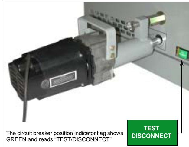
Figure 6: ERD Mounted on the Circuit Breaker Compartment Door (Circuit Breaker in the TEST/DISCONNECT Position)
