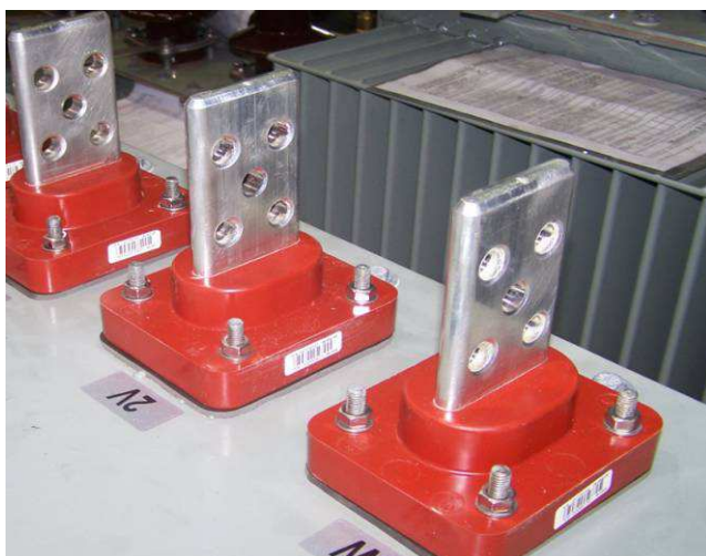
Fig. 8. LV bushings type „busbar” according to EN 50387:2009
