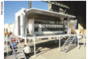
Self-standing primary MV/MV substation with side opening walls, allowing additional space of operation
