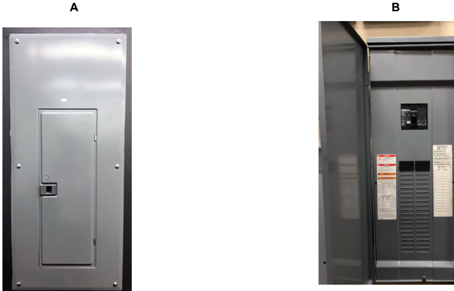
Figure 4 – Indoor and Outdoor Load Centers (Examples)
