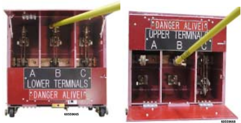
Figure 8: Placing Selector Switches In the Closed Position for Grounding Using a Hookstick—Upper and Lower Shown
