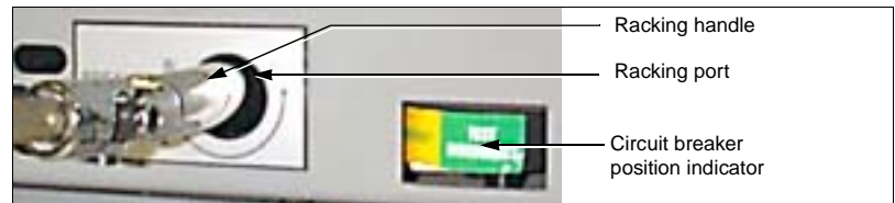
Figure 7: Racking Handle Engaged onto Racking Shaft with Circuit Breaker in the TEST/DISCONNECT Position
