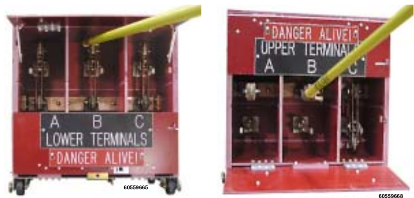
Figure 10: Closing Selector Switches (for Grounding) with a Hookstick—Upper (left) and Lower (right) shown
