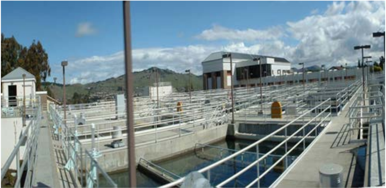
Vallejo Water/Wastewater facility
