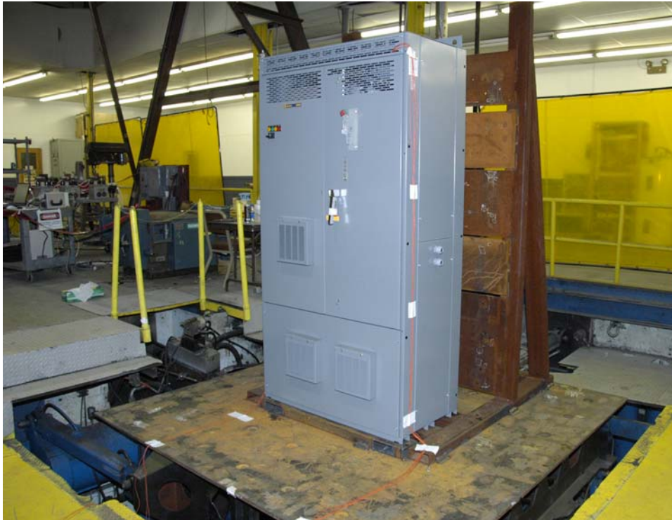
Figure 2: 18-Pulse Device Mounted to Test Stand at Wyle Labs
