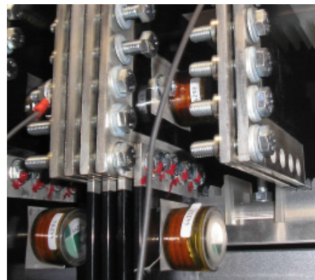
Photo shows the placement of temperature monitor sensors attached to service entrance bussing.
