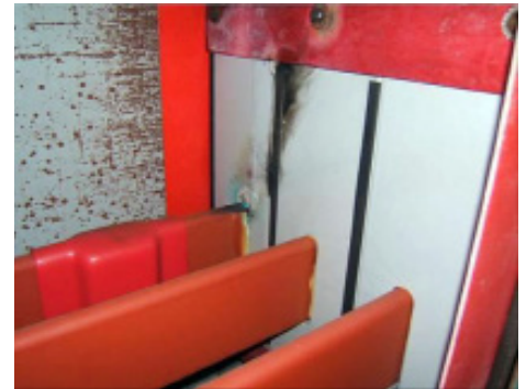
Photo shows clear indications of corona tracking due to damaged insulation laminate on bussing and long term electron tracking prior to a phase-to-ground fault condition.
