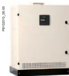
Cubicle A2 with incoming circuit breaker.
