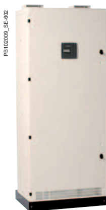
Cubicles A3 and A4 with incoming circuit breaker.
