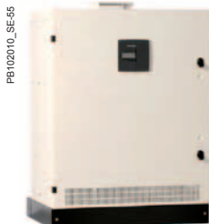
Cubicle A2 with incoming circuit breaker.
