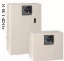
Enclosures C1 and C2 without incoming circuit breaker.
