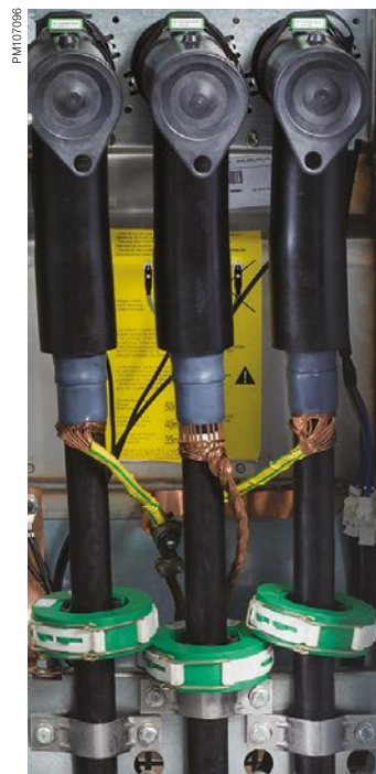
Current sensors mounted at site around single core cables
