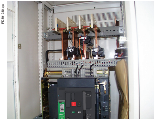
CT on vertical busbars.
