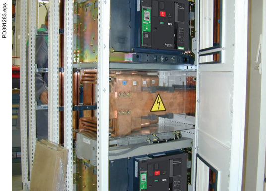
Source changeover system in the same cubicle.
