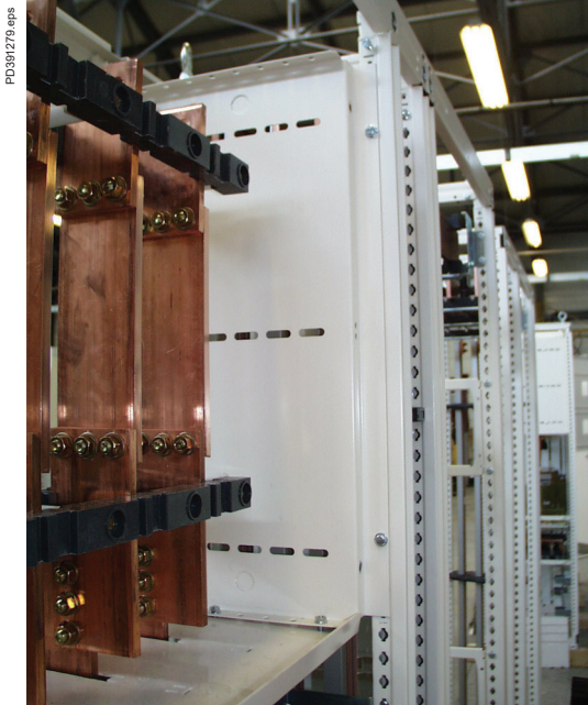
Dismountable vertical busbars.
