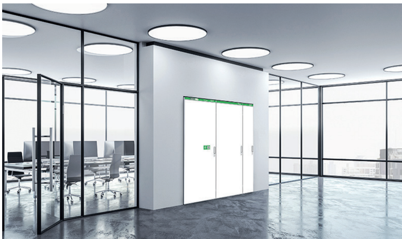
PrismaSeT Active wireless panel server installed into its environment
