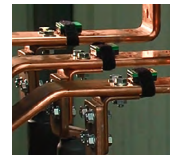
Set of Easergy TH110 sensors fixed on the 3 phases of an electrical connection
