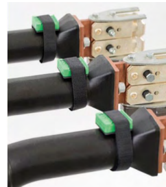
Connection temperature monitoring
