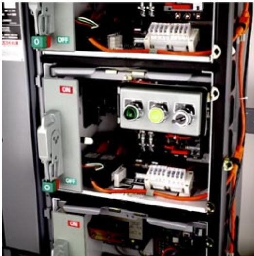
MCC Starter Unit with SERIPLEX Discrete I/O Module (Terminal Blocks Not Required)
