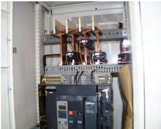
CT on vertical busbars.
