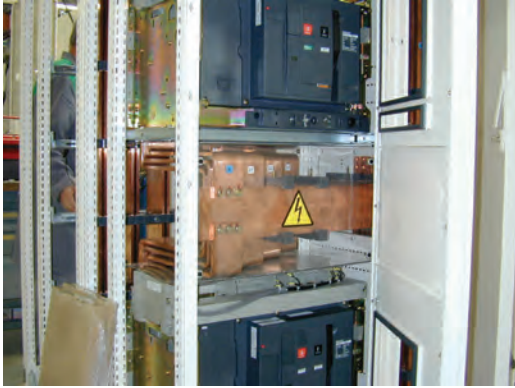
Source changeover system in the same cubicle.
