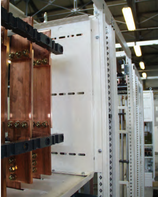
Dismountable vertical busbars.
