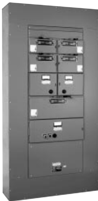
QMB Motor Starter Center with Fusible Disconnects
