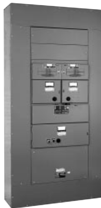
QMB Motor Starter Center with Circuit Breaker Disconnects
