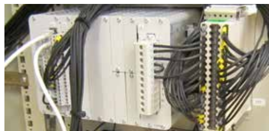
Arc protection systems require three phase currents for selective high-speed arc protection. Using the zero-sequence voltage and current in tripping criteria, the arc fault trip can be activated before the fault is completely exposed.
