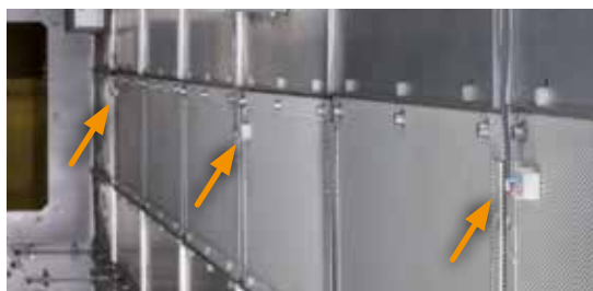
Point sensors are mounted in the switchgear's arc pressure relief compartment in this installation.
