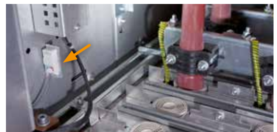
The majority of arc faults occur in the cable compartment hence it is a natural location for the point sensor.
