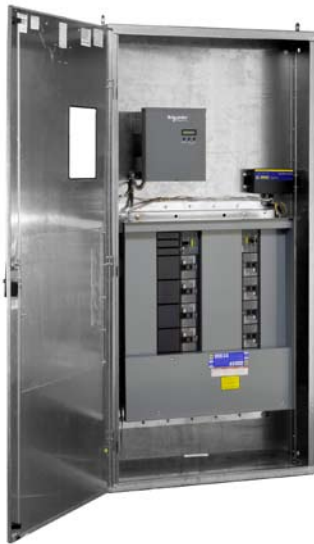
PowerLogic EM4800 meter shown embedded within a power distribution panel.
