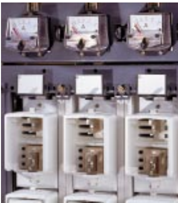
Load monitoring of outgoing circuits
