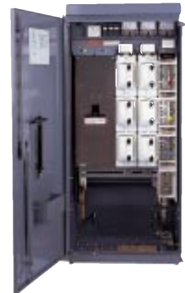
Fuse cabinet with 2 x 630A Shielded fuseways and up to 1250A outgoing mccb.
