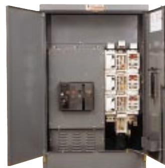
Flexible supply for larger ratings, combine acb and Shielded fuseways within a Feeder Pillar.
