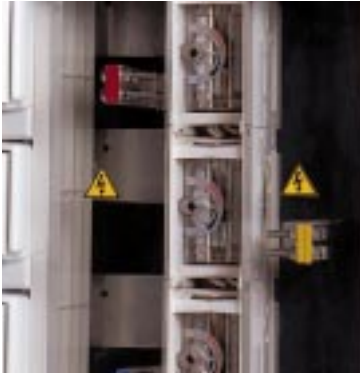
Padlocking device fitted to incoming disconnector
