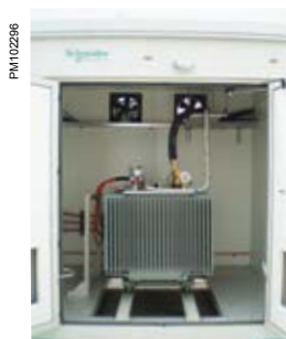
Transformer in PV box
