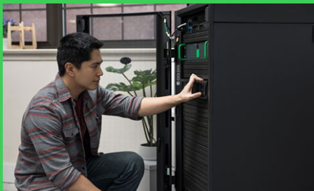
Micro Data Center
