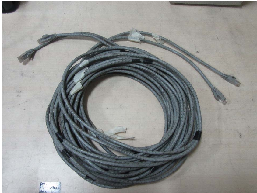
Figure 34: Photograph of NMC Ethernet cable
