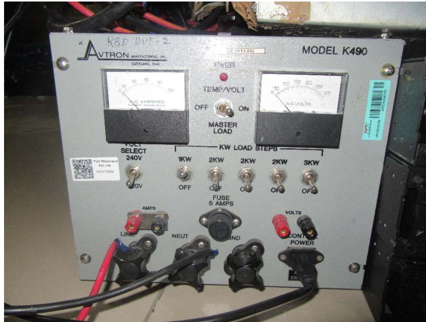
Figure 31: Photograph of resistive load
