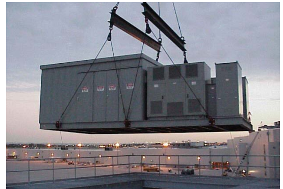
Two substations with PZC base extension
