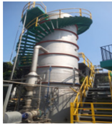
Zero Liquid discharge plant in SLW, Kolkata.
