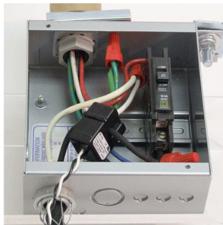
Figure 2. CT connected to circuit for a busway tap box installation
