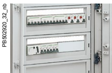
Detail from the Circuit Marking System
