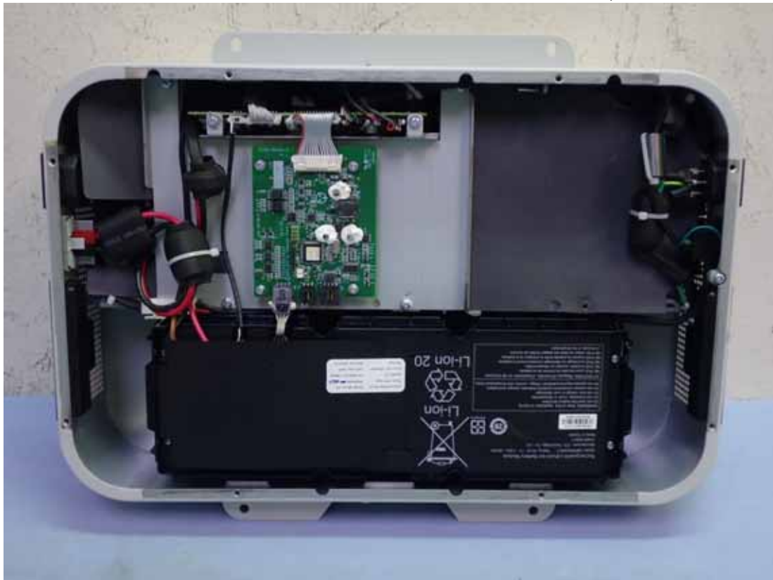
Figure 7 Internal View (Removed Covers)
