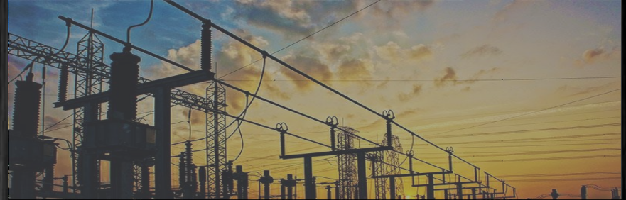
Powering Andhra Pradesh's Future with Substation Supply
