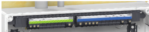
Modular terminal blocks with screwless quick connections for small cables - earth and neutral terminal blocks
