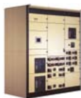
LV Switchboard Okken
