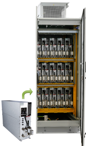
Fig. Power cells cabinet and Power cell
