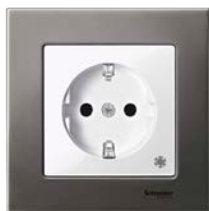
Socket-outlet marked freezer
