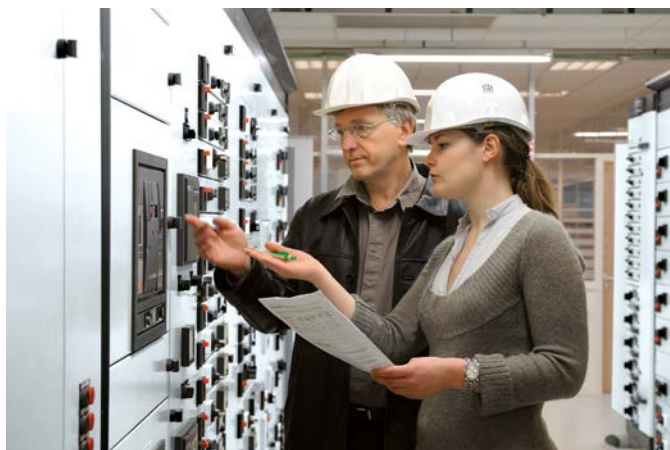
Quadro Motor Control Centre (MCC).
