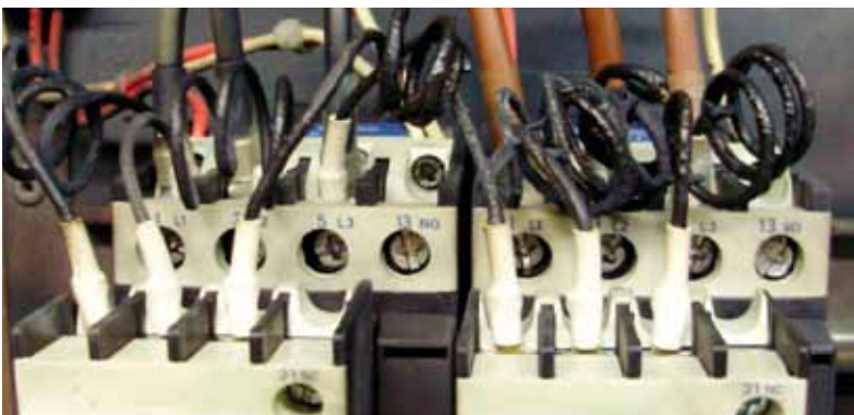
Example of damaged damping resistors
