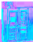
LV Switchboard Prisma
