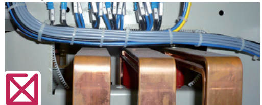
The cables are routed too close to the power bars.
