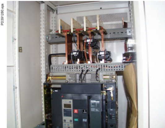
CT on vertical busbars.
