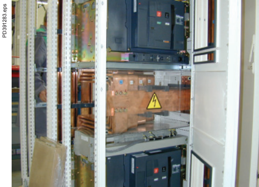
Source changeover system in the same cubicle.
