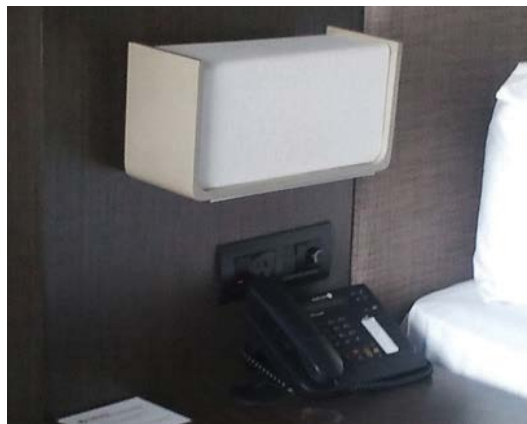
Modena power outlet and dimmer
