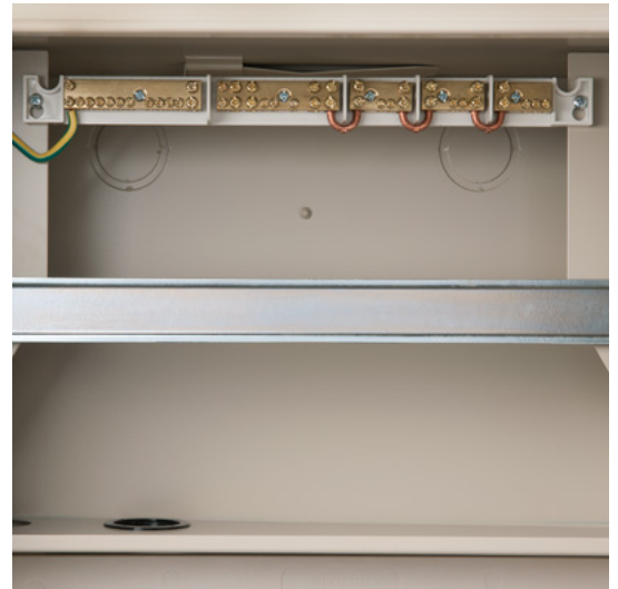
Generous wiring room and well-located cable knockouts
