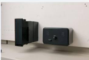
Service fuse holder and neutral link
