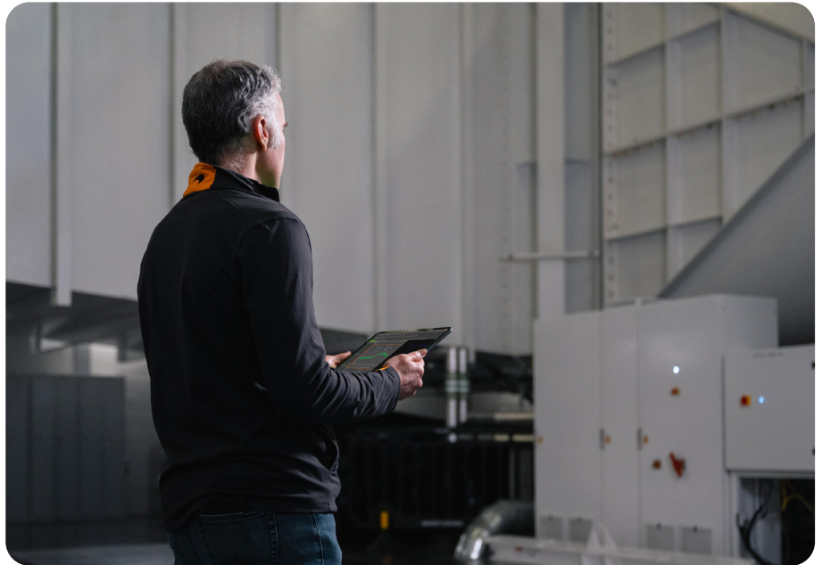
EcoStruxure Power Monitoring Expert works with the MTC’s existing infrastructure.
