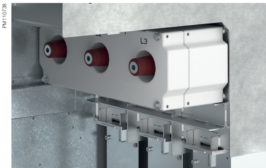
Current transformer block on bushings with optional supplementary core, cubicle width 600 mm
