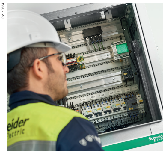
Low Voltage cabinet
