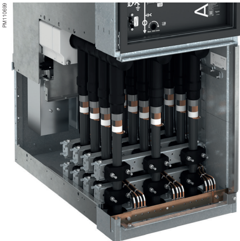
2 cable fixing iron supports for cables with cross section \geq 500 \text{ mm}^2
