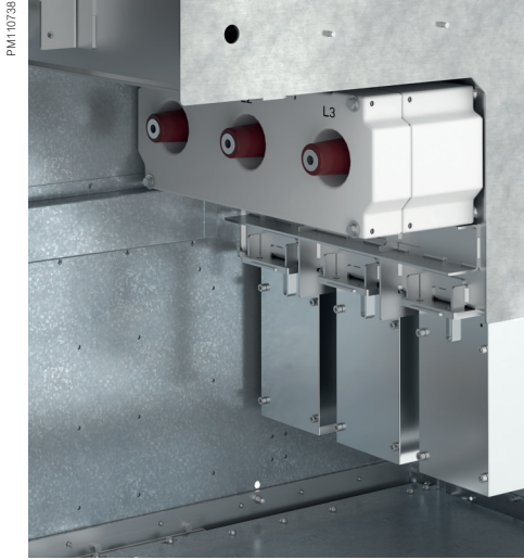
Voltage transformer in cable compartment with disconnecting device
