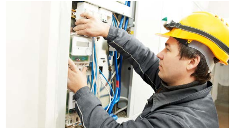
California's Title 24, Section 130.5(a) requires all mandated capabilities be incorporated into a single meter for the largest energy users.
