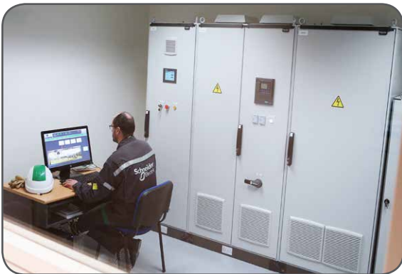
A Schneider Electric technician analyses the performance of the integrated power conversion and battery storage system.
