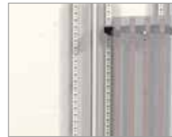
Lateral busbars. The bars are staggered for easy access to connection points.
