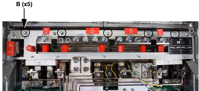
Figure 46: Top Terminal Bracket Bus Bar Connections
