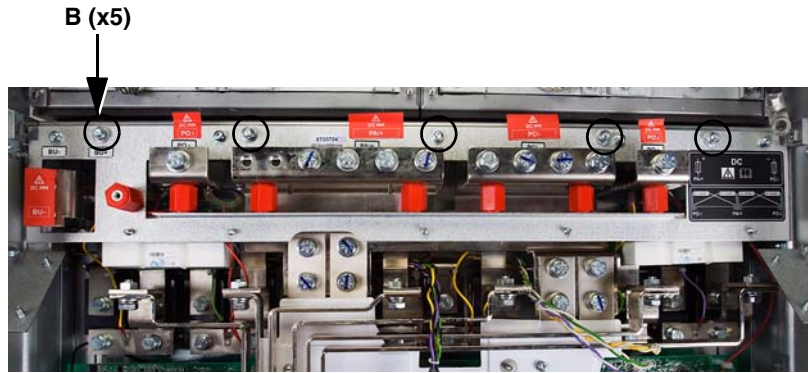
Figure 177: Top Terminal Bracket Bus Bar Connections
